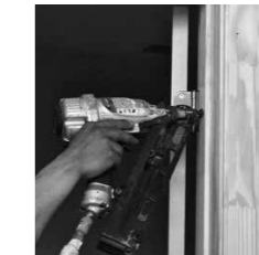
Door frames drilled and anchor bolted to the brick wall to provide better strength and durability
