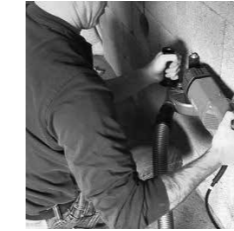
Electrical conduits cut by a machine and debris scooped out by a scooper instead of using a hammer and chisel to reduce stress on bricks and avoid cracks
