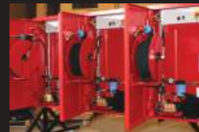
Modern Fire Fighting System
