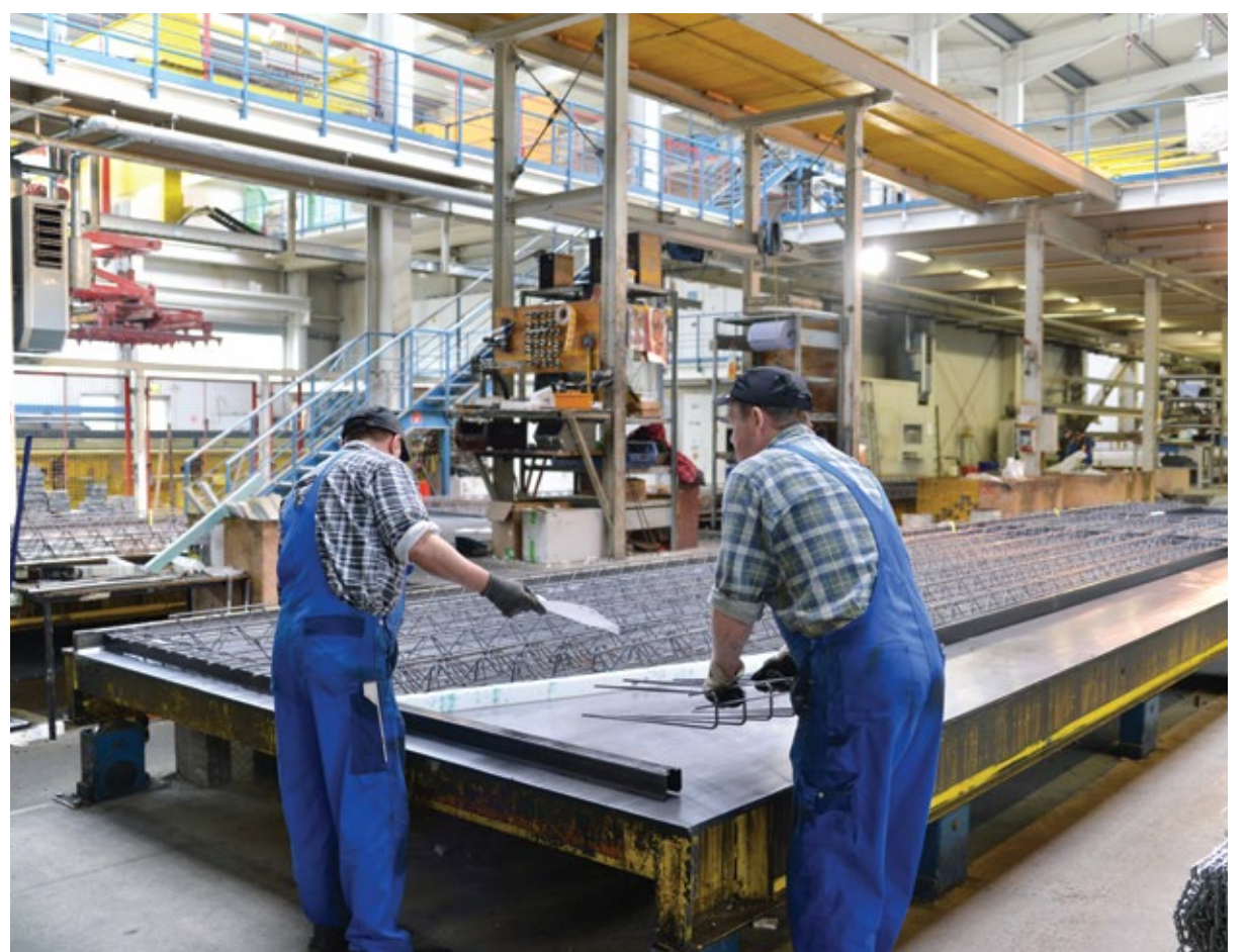
Precast Facility Spread Across 73,000 sq. ft.
