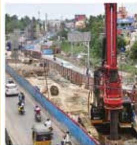
Working ahead Metro rail work in full swing at Kilambakkam on the Madhavaram-Sripuram line, which is proposed to be extended till Kilambakkam. -G. Subramanian/ANI
