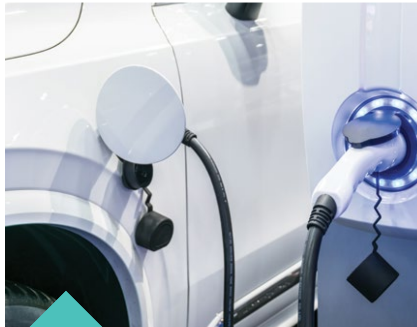
Individual car charging point in each car park so that you can charge your EVs with ease. A separate sub-meter is also provided for you to track your power consumption.
