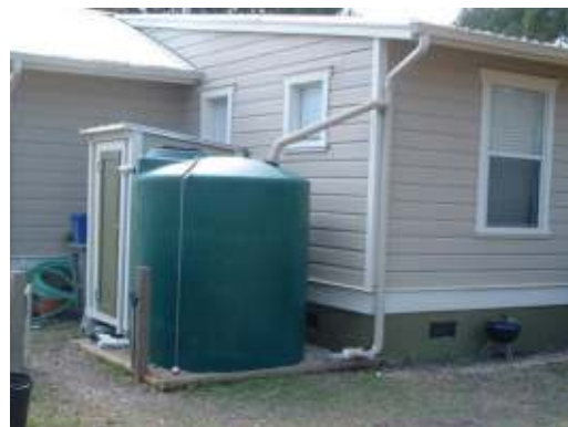
RAIN WATER HARVESTING
