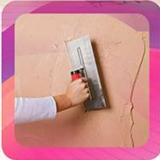
PLASTERING All internal walls smoothly plastered with lime rendering and double coat sponge finish for external walls.
