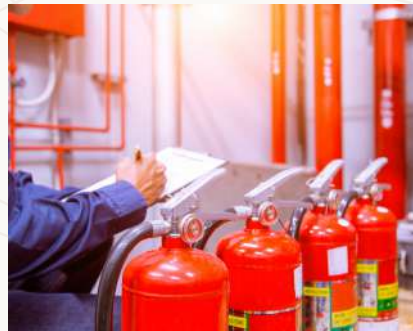
Fire fighting System
