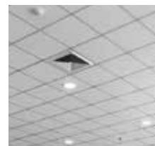
CEILING GRID FALSE CEILING
