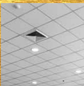
CEILING GRID FALSE CEILING
