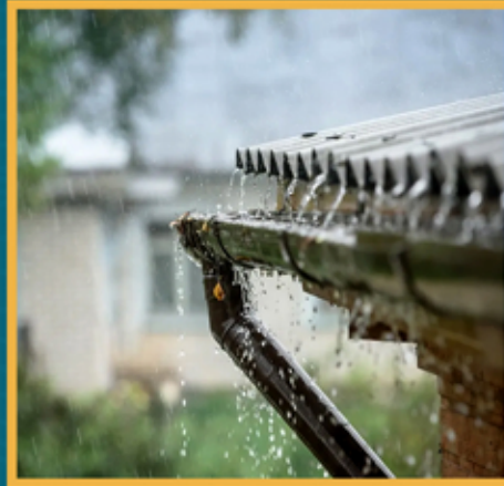
Rainwater Harvesting System
