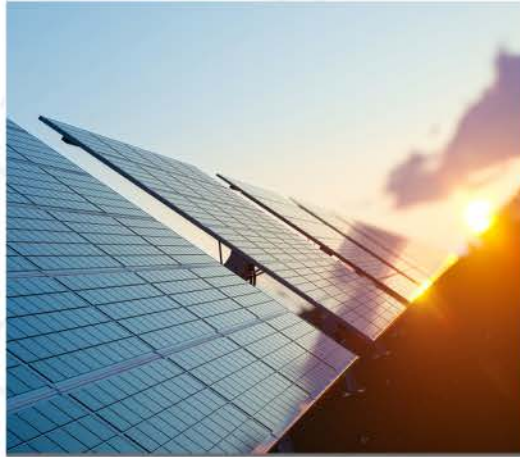
Rooftop Solar PV Systems
