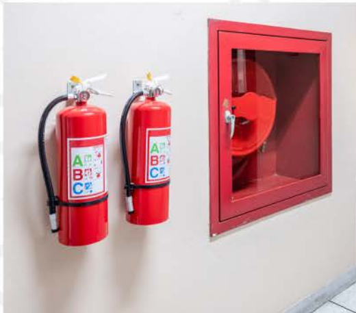
Firefighting Systems With All Fittings With ISI Marking
