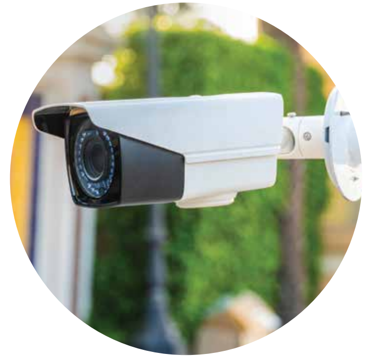
CCTV Surveillance in Main Entrance for Each Wing
