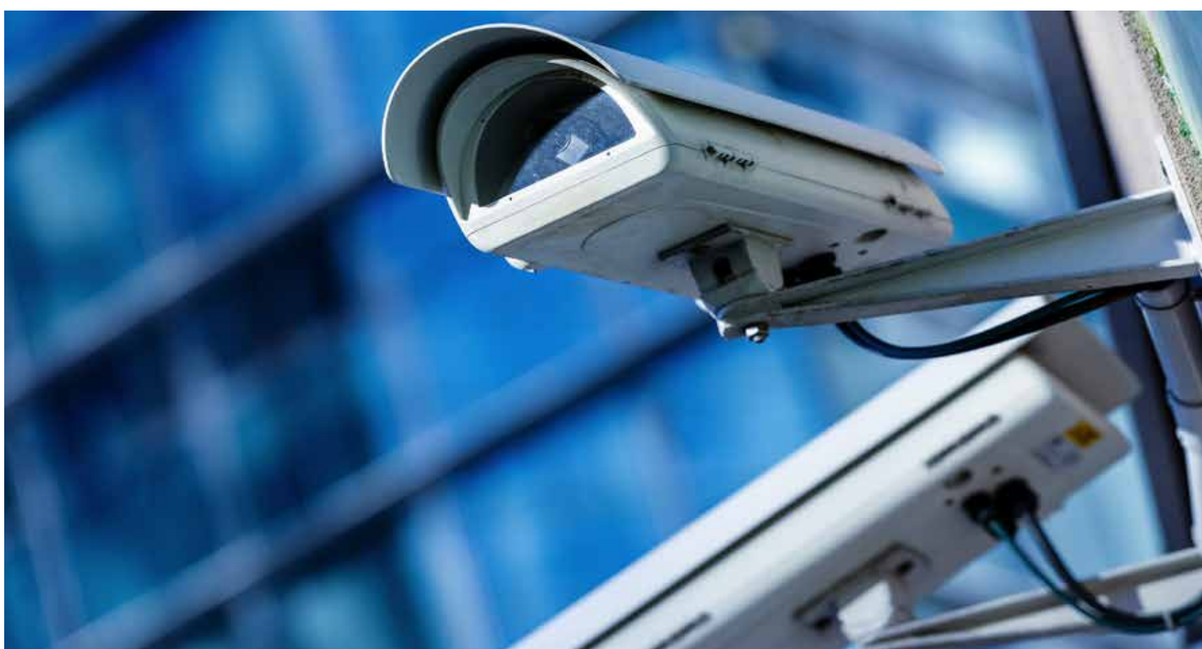
CCTV CAMERA SURVEILLANCE
