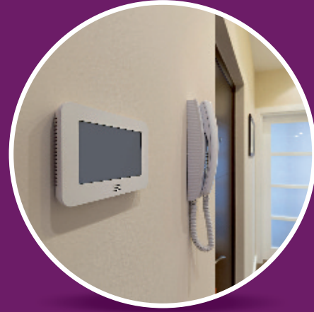
VIDEO DOOR ACCESS AT LOBBY
