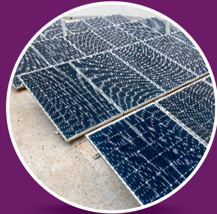
SOLAR POWER (Common Area)
