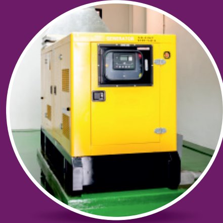
GENERATOR BACKUP (Common Area + Partially For Apartments)
