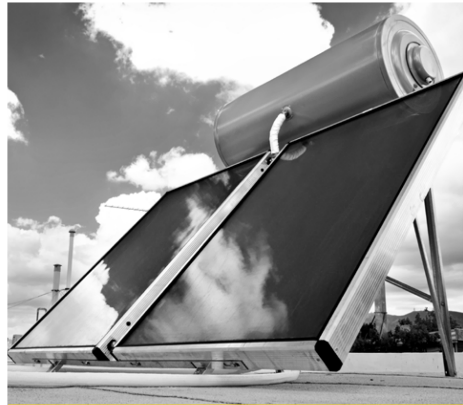
SOLAR WATER HEATING
