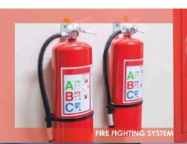
FIRE FIGHTING SYSTEM
