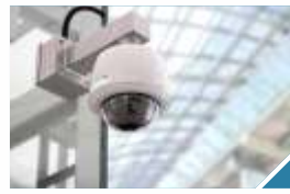
CCTV CAMERA SYSTEM
