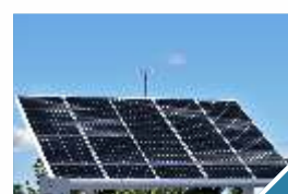
SOLAR PANEL SYSTEM
