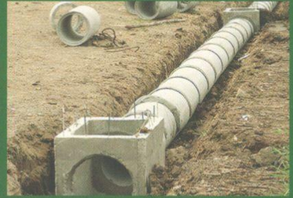
Strom Water Line
