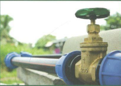
Drinking Water Line
