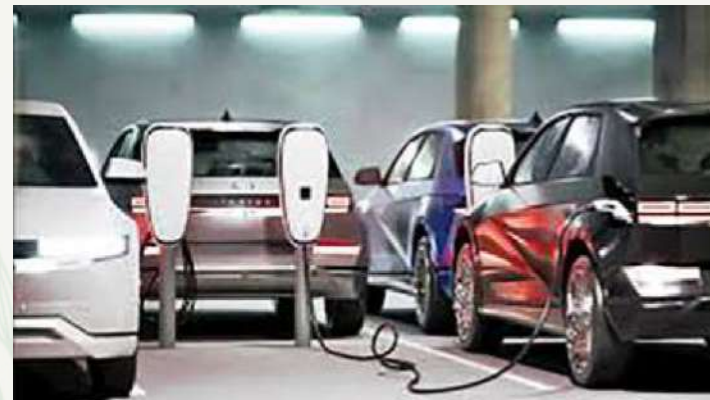
COVERED CAR PARKING WITH EV POINTS
