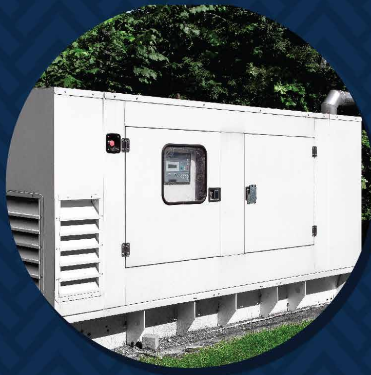
POWER BACK UP FOR COMMON AREA & FLATS
