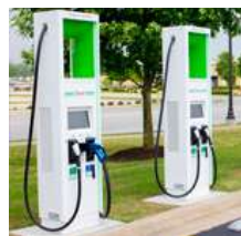
EV CHARGING STATION
