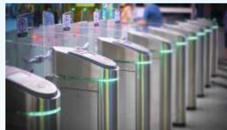
Access control system
