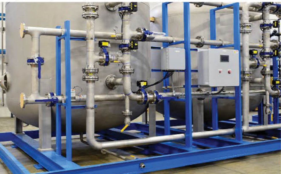
Water Softening Plant
